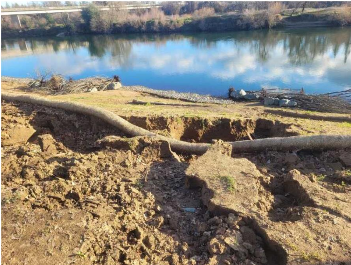
Photos of new soil covered revetments and planting benches blown out after recent rains. This wouldn't have happened if natural vegetative armoring had been left intact.
